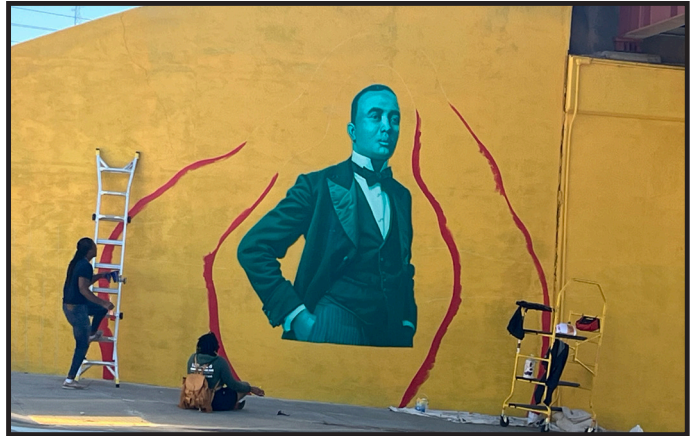
Installation of Pathway to Hope Public Art Trail: Visionaries by Alexander Tamahn and Joel Daniel Phillips, Oklahoma Art in Public Places
